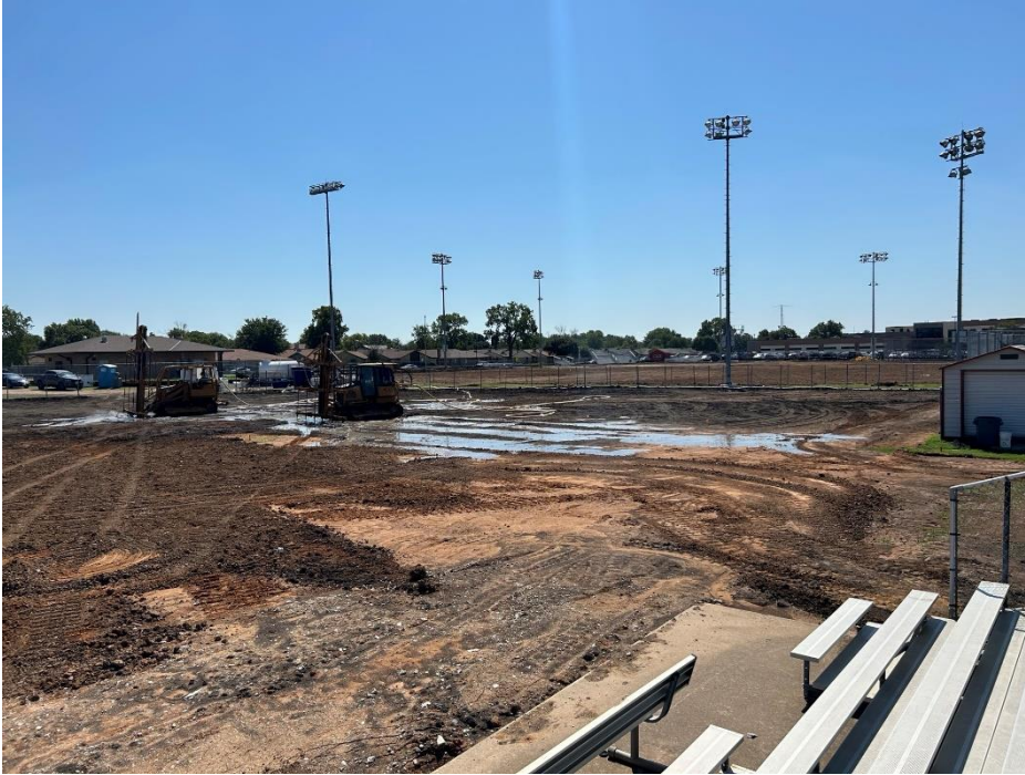
North Garland, Chemical injection at Softball Field
