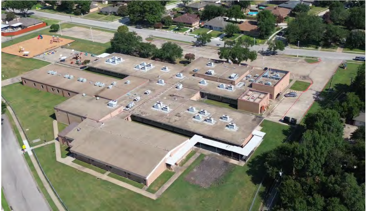
Paragon Roofing and LBL are working with GISD Maintenance to make sure roof-top units are disconnected and removed safely and remain intact.
